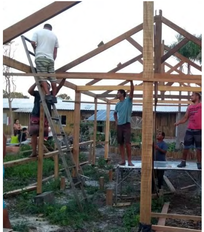
Community members build a house in Nova Enseada, their chosen relocation site. © Carolina Kotchetkoff, 2017
